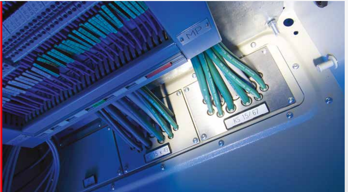
KDP 105/15 in the control cabinet
