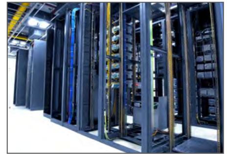
Servers, routers, switches, data centers and more
