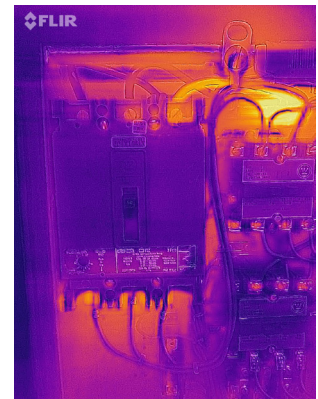
Identify electrical faults
